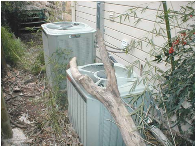
Condenser Units (left side)
