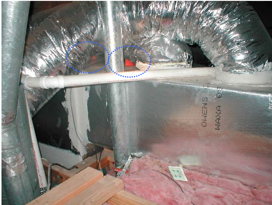
Variable Air Volume Dampers (motor actuators are the orange boxes)
