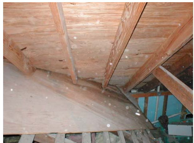
View beneath Left Valley (lots of leakage)
