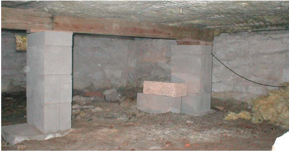
Inadequate Shaker Supports (dry-stack CMU)
