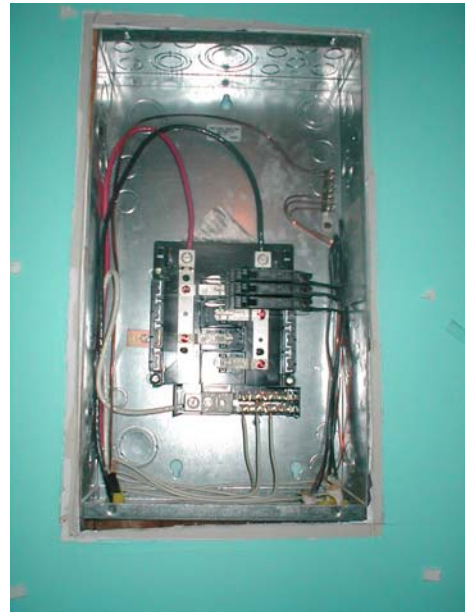
Interior Subpanel (upper bedroom)
