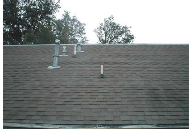
This Area (right rear, facing west) Appears Hail-Damaged
