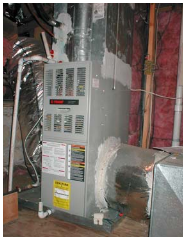
Lower (main) Fan-Coil-Furnace
