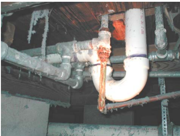
View of Galvanically Incompatible Supply Connection (leaking)
