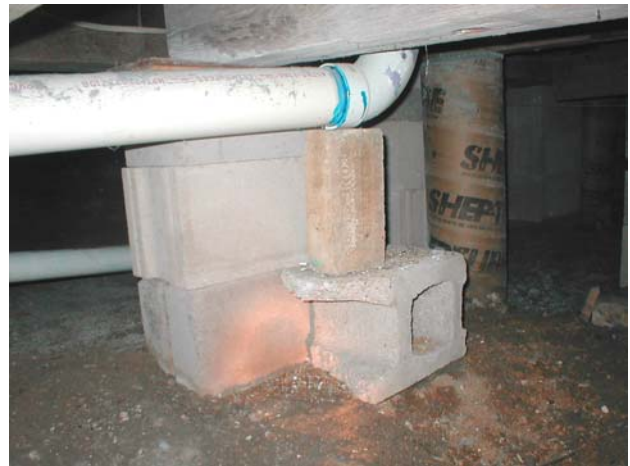
Improvised Piping Support (utility branch)
