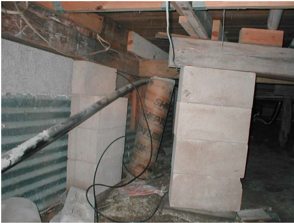
View at Rear Crawlspace (upset sonotube, dry-stack shoring, 'ad-hoc' cribbing, etc.)
