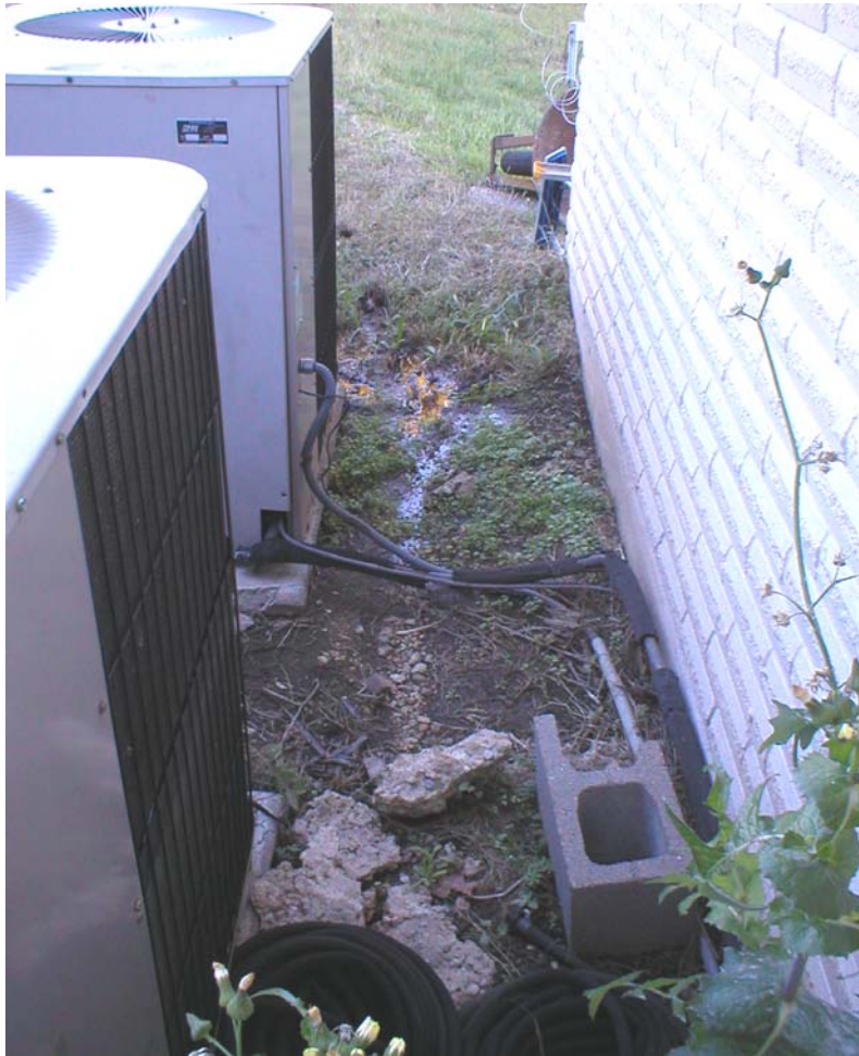
Standing Water Upslope of Foundation (rear, to right of driveway)
