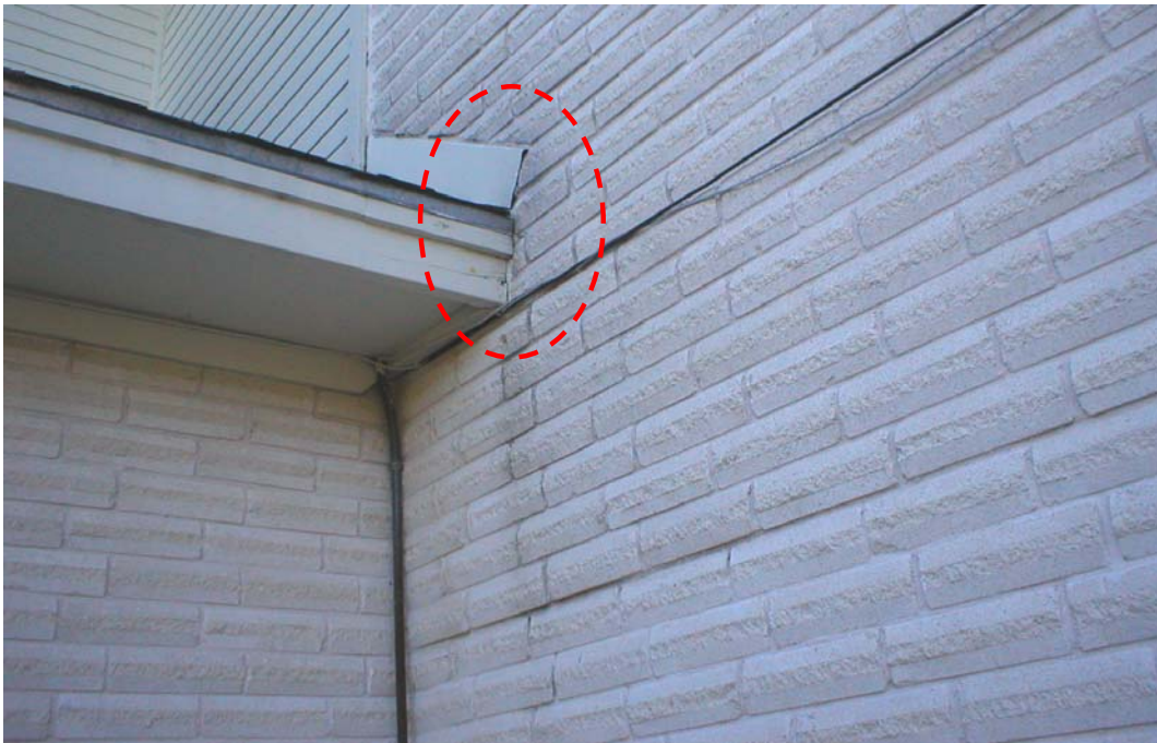
Example of Inadequate Roll Flashing with No Kick-Out (one of several)
