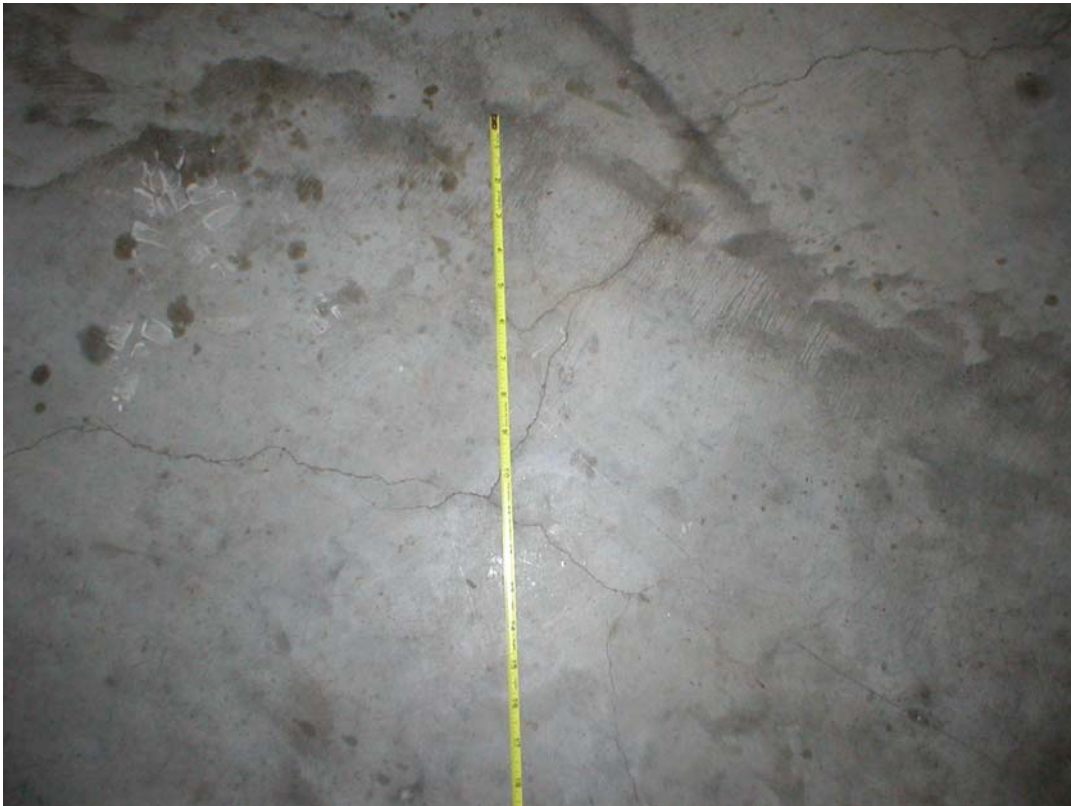
Shrinkage Cracks at Garage Floor
