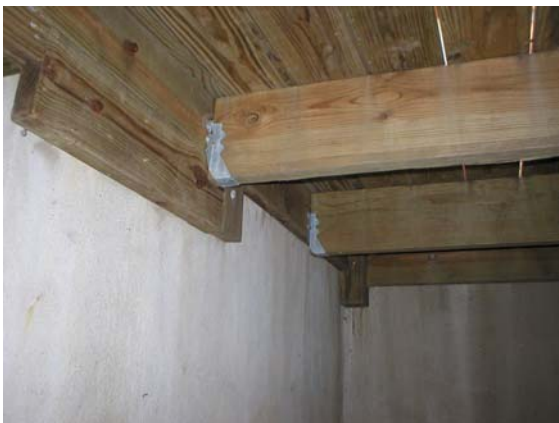
Under-Sized Joist Hangers, Inadequate Lags (beneath deck)
