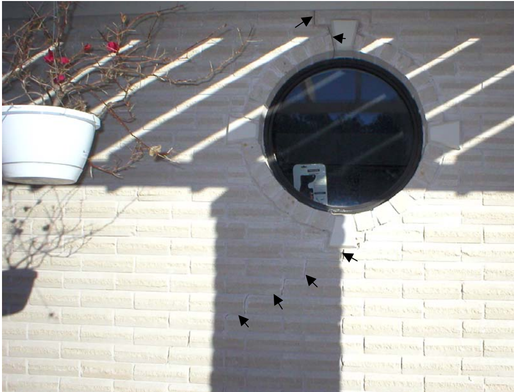
Flexural Crack at Front Elevation (left of entry)
