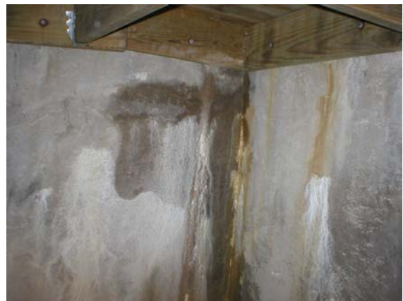
Seepage at Pool Enclosure (beneath deck, near spa)
