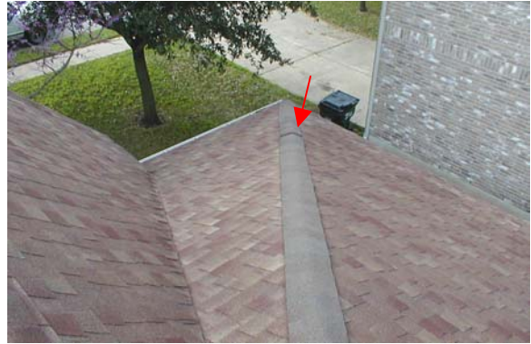
Missing Ridge Tab (front left hip)
