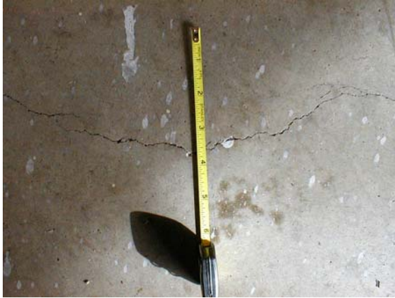
Slab Shrinkage Crack (at garage)
