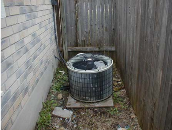
Exterior Cooling Equipment (left side)
