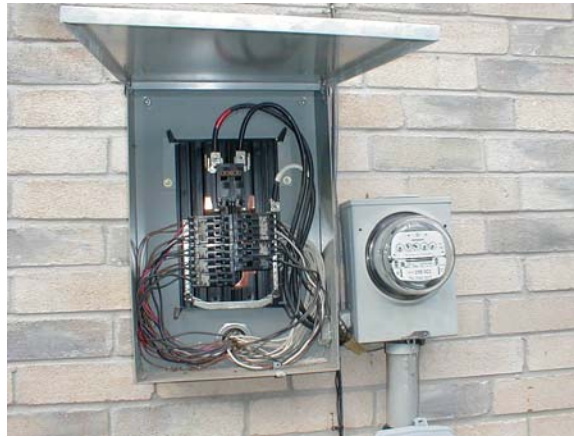
Exterior Service Entrance and Distribution Panel (right side)
