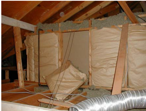
Fallen Batting at Attic (raised ceiling walls)
