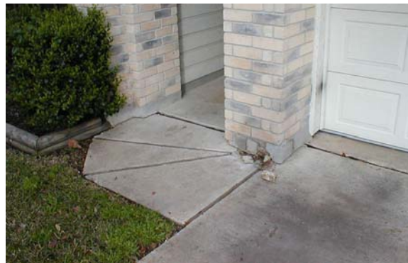
Front Masonry Veneer over Flatwork Slip Joints
