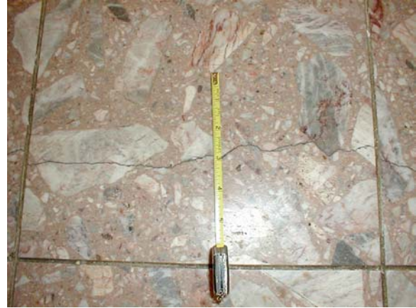
Reflected Shrinkage Crack (at foyer)
