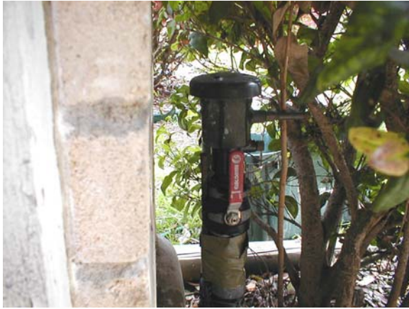
Sprinkler Anti-Siphon Valve (leaking)
