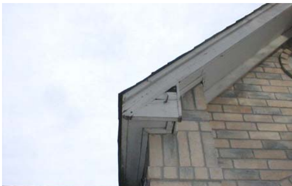
Deteriorated Fascia & Eave Trim (front)
