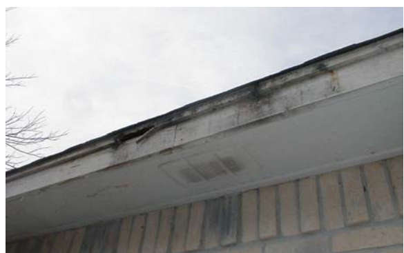
Deteriorated Fascia and Drip Mold (right)
