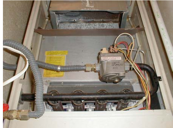
Furnace-Fan-Coil (at foyer mechanical closet)
