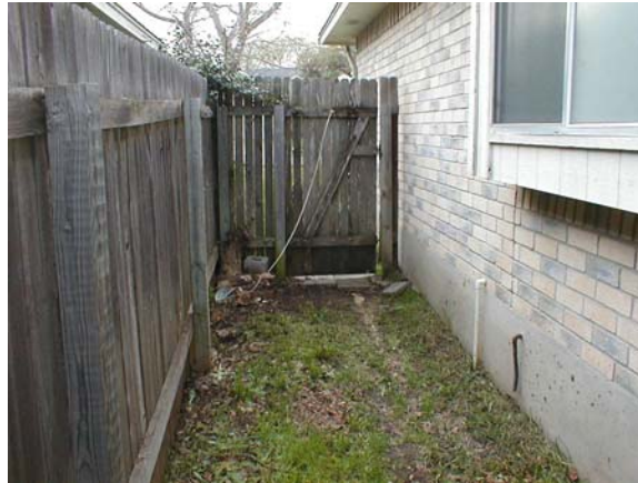
View of Right Yard (progressive erosion beneath eave)
